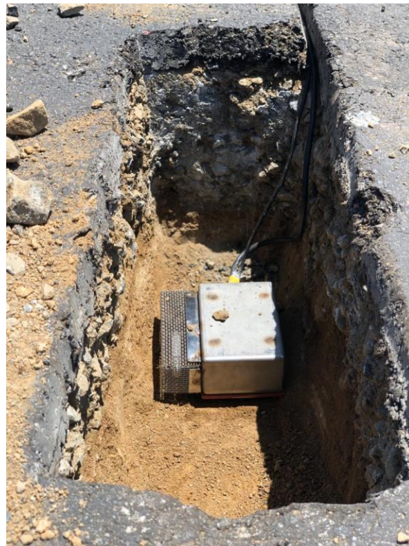
Figure 4.0: Sensor embedded into road pavement
