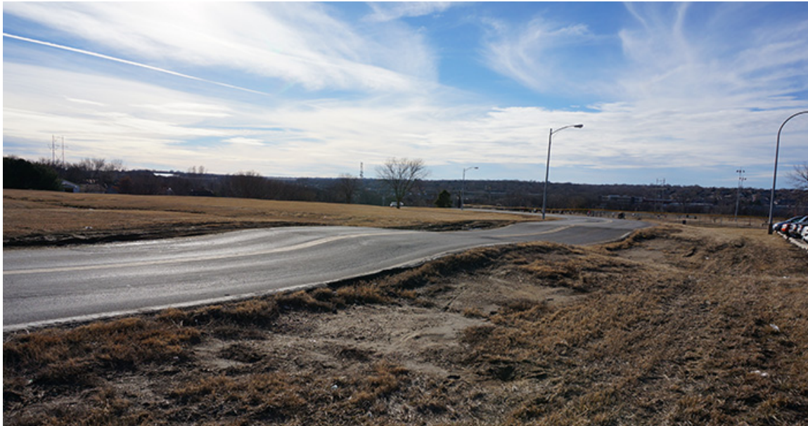
Figure 15: View of road in Heflinger Park looking southwest of where it crosses two of the trenches with waste fill that underwent significant compaction during biodegradation. The road has since been regraded and repaved, but additional subsidence continues.
