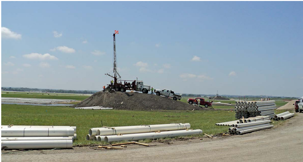
Figure 29: One of the drilling sites during the 2011 flood Eppley airfield dewatering response. The levee and river are to the viewer's back. Note how the drill rig had to be on an elevated pad. To the left of the drill pad is one of the seep sites with a gravel pad installed on top to stabilize the sediment and prevent liquefaction and attendant loss of strength. Photograph courtesy of Griffin Dewatering.
