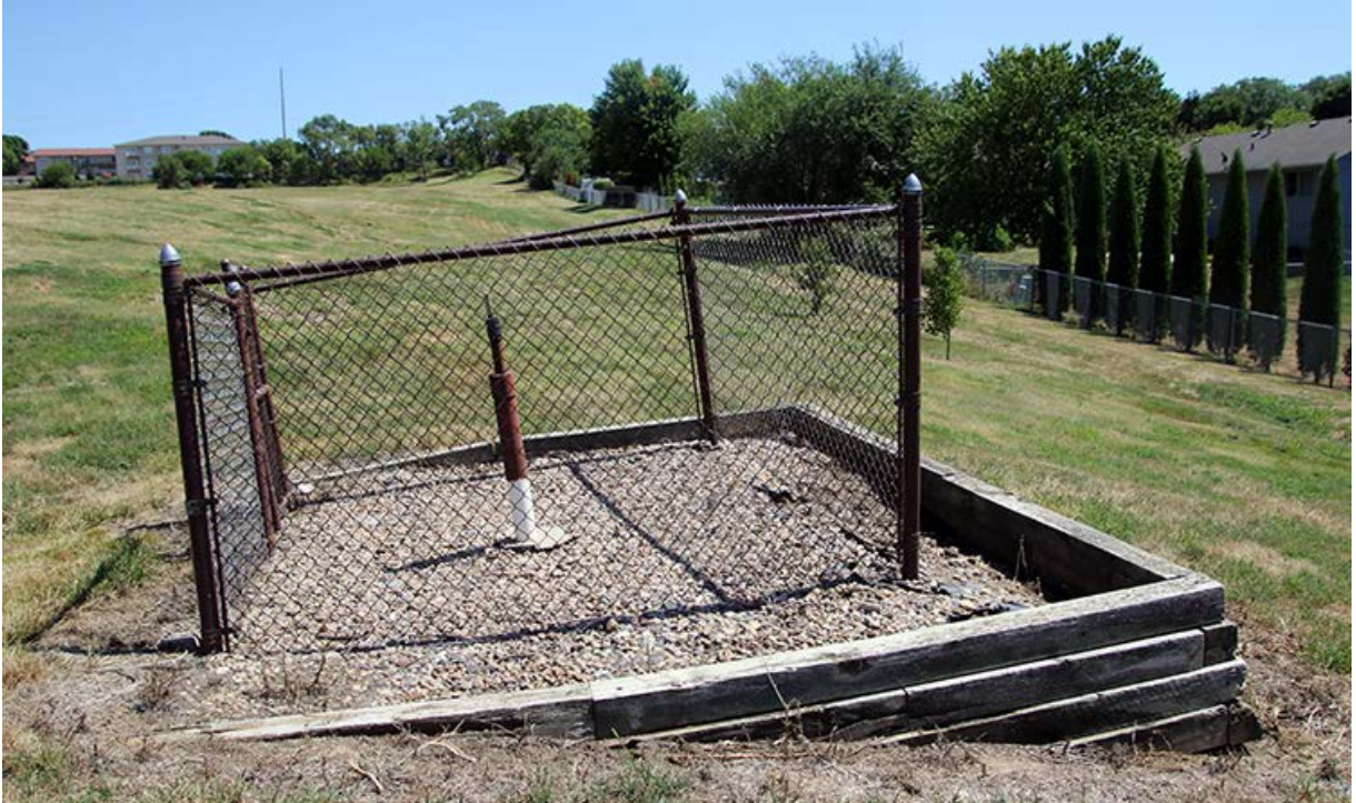
Figure 17: View looking east at uppermost methane venting site. A sign on the gate says “no smoking”. In the upper right image section a small drainage ditch, along with a house belonging to the development to the south, also is evident. Image taken in August 2022.
