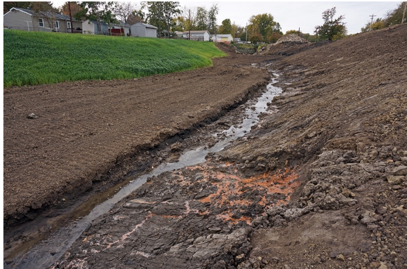
Figure 38: Image taken during construction associated with the restoration project (Oct. 2015). The intentional channel meanders are evident. Some of the bank material was clay and organic
