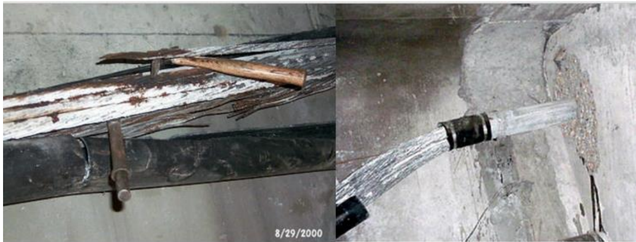
Figure 6: Tendon failures on the Mid-Bay Bridge (FDOT, 2002)
