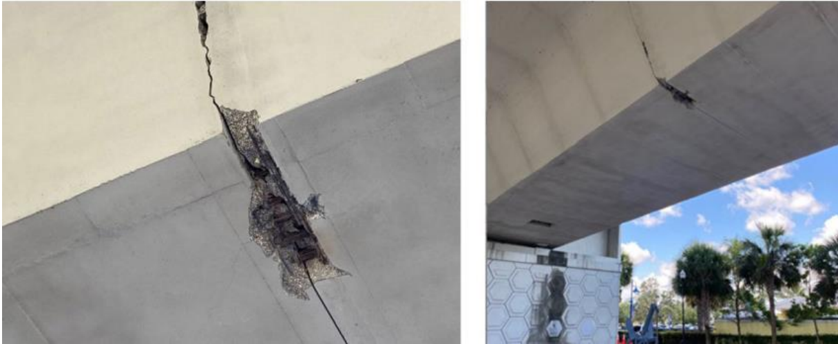
Figure 13: Localized corrosion damage for internal tendon in Stuart, FL (Roustan and Erblat, 2020 & Detman and Rodriguez, 2020)
