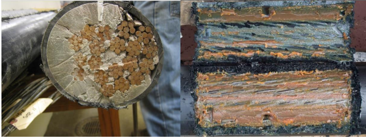
Figure 4: Duct filled with CG (Left) (FHWA, 2014), Duct filled with FF (Right) (Hamilton et al. 2017)
