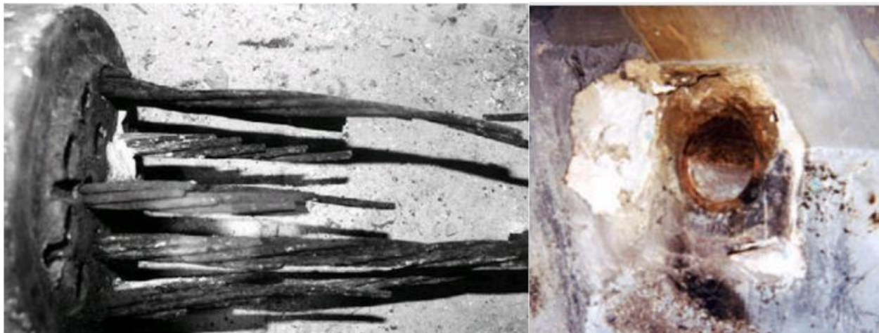
Figure 5: Corrosion of strands in the anchorage (Left), Anchorage of the Failed Tendon with Water Staining from the Leaking Expansion Joint (Right) (FDOT, 2002)
