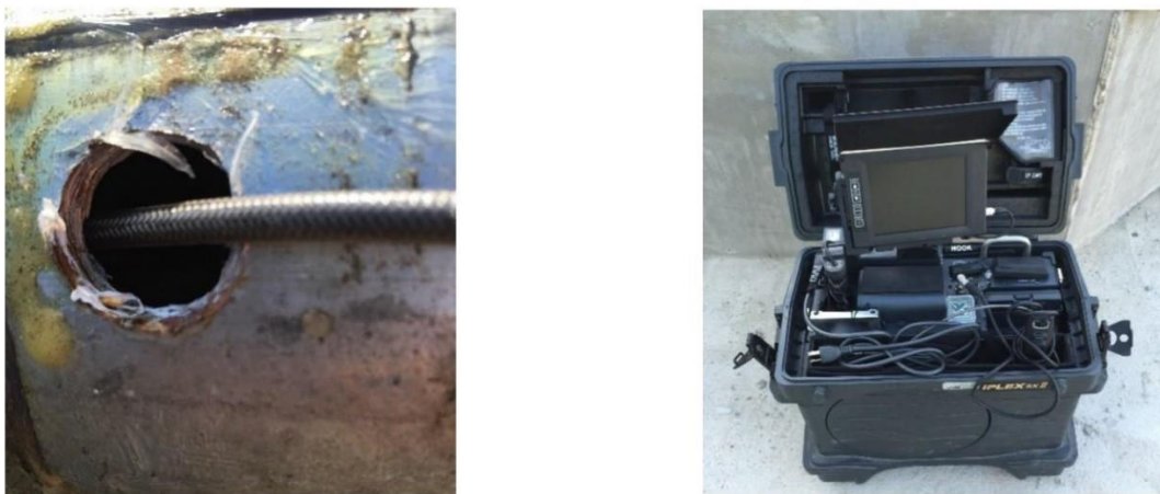
Figure 124: Depicts the borescope access port and the equipment used (Hurlebaus, Hueste, Karthik, and Terzioglu, 2016)
