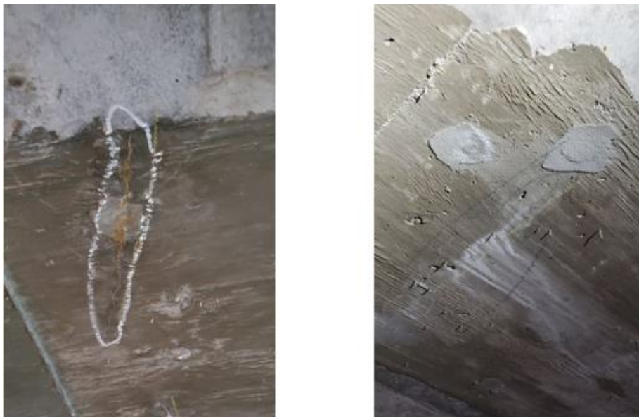
Figure 15: Example of cracking (Left) and efflorescence (Right) from the eastbound Seabreeze Bridge Inspection
