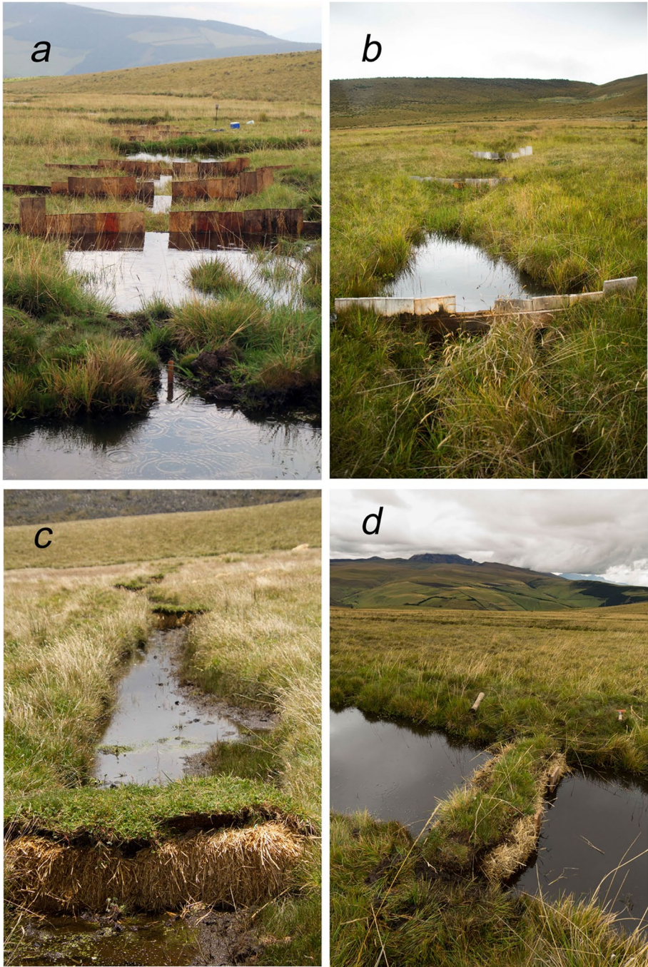
Fig. 5 Examples of the barriers constructed with wood planks ( a and b ) or straw bales ( c and d ) to slow down water movement along the ditches, and promote rewetting in the Chakana peatland
