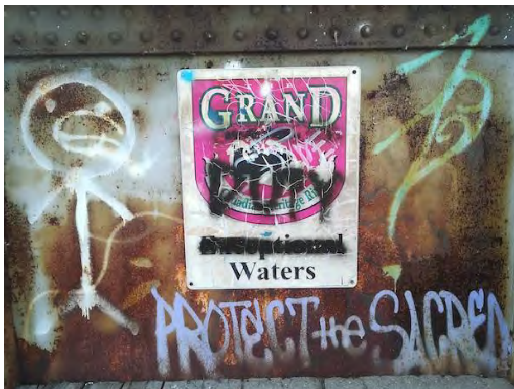
Figure 7. Train bridge crossing over the Grand River, Brantford, Ontario. Photo by Sarah Van Borek (2018).
