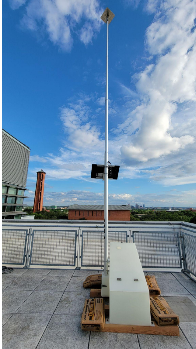
Figure 2.1.A. Front view of the Emergency Water Station 3.0 device on the roof of the CSI building at Trinity University.
