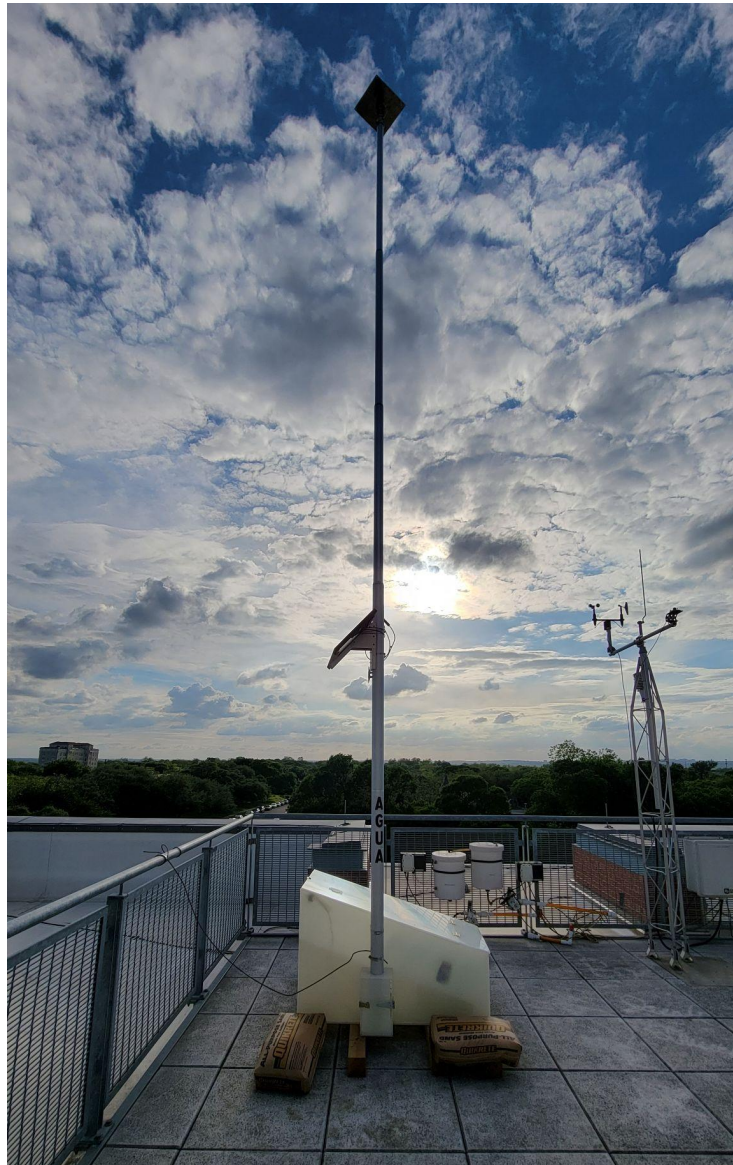
Figure 3.8.B. Emergency Water Station 3.0 device installed on the fifth floor roof of CSI for the Wind Stability and Weatherproofing Field Test. Note that we grounded the station using a wire attached to CSI railing which was grounded.
