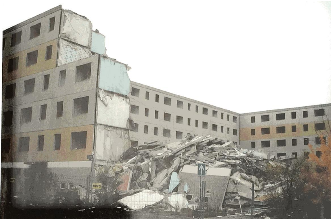
Figure 6.4 Photograph of the demolition process in the southern portion of WK VII , ca. 2003-2004. Source: Peter Ullrich and Gabriele Haubold, “Stadtumbau aus Gesamtstädtischer Perspektive,” Stadtspiegel (June/July 2004).
