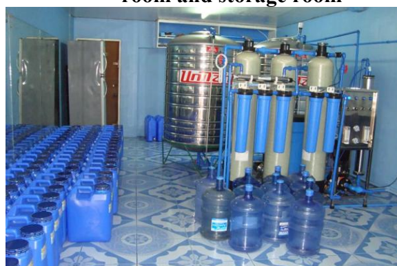
Figure A6.1a: Enclosed water purification room
