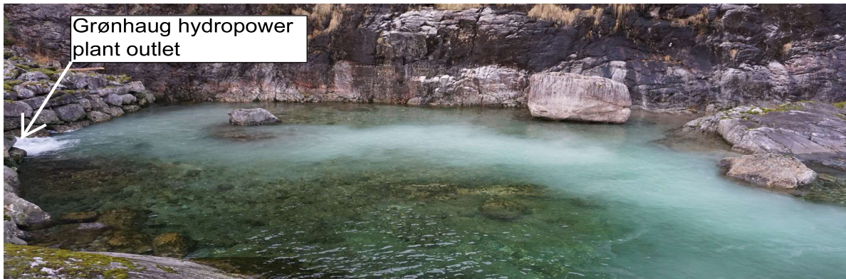
Figure 5.4: Grønhaug plant outlet river during field third covering of intake trash rack at field tests the 26th of November
