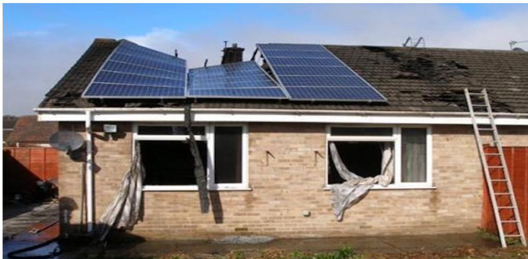
Fig 2.2 Destroyed rooftop solar power plant near the city of Irpin (Kyiv region) [8]
