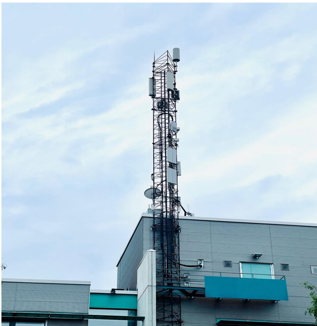
Figure 42. 5G New Radio BTS of 5GTN at the University of Oulu (Linnanmaa campus) on existing infrastructure.
