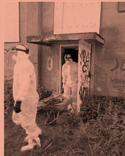
△ Fig 49. More than 5 containers of trash were taken out of the silo
