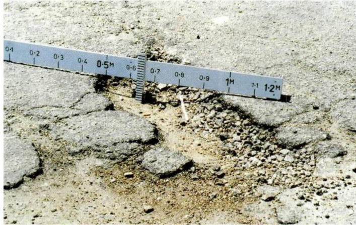
Figure 6.3: Example of pavement surface texture deficiencies - pothole (adapted from Research & Development division of the Highway Department (2013) ).
