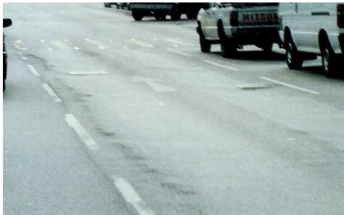
Figure 6.2: Example of pavement deformation - rutting (adapted from Research & Development division of the Highway Department (2013)).
