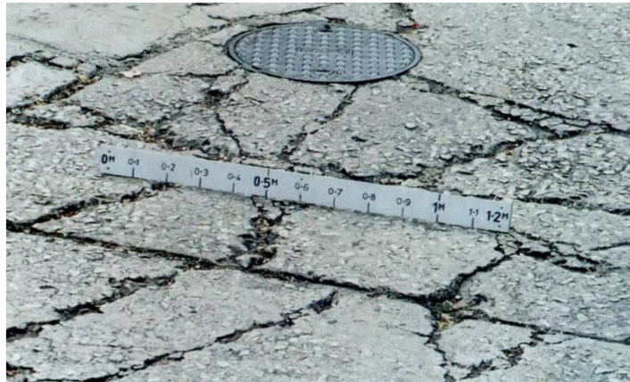
Figure 6.1: Example of pavement cracking (adapted from Research & Development division of the Highway Department (2013)).
