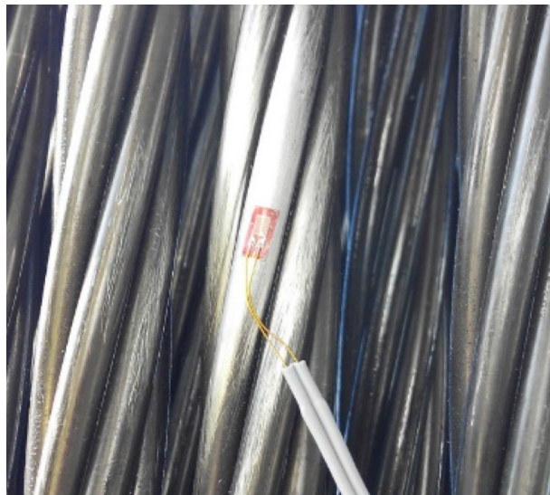
Figure 6. Installation of unidirectional strain gauges on one of the wires of a strand in a temporary cable.
