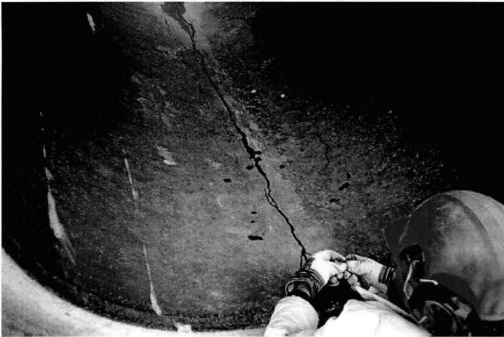
Figure B-26. Crack Formed at the Inner Surface of the Pipe
