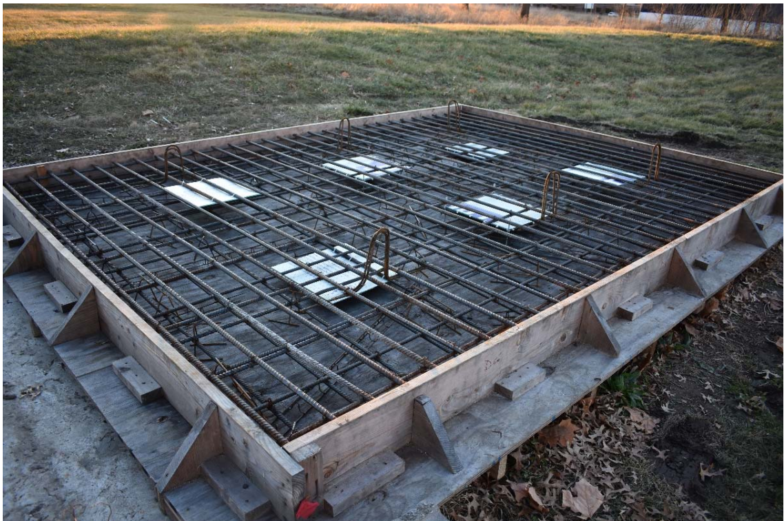
Figure 4-6: Details of both layers of steel reinforcement, top and bottom, the locations of defects, and locations of hooks in the specimen before pouring the concrete.
