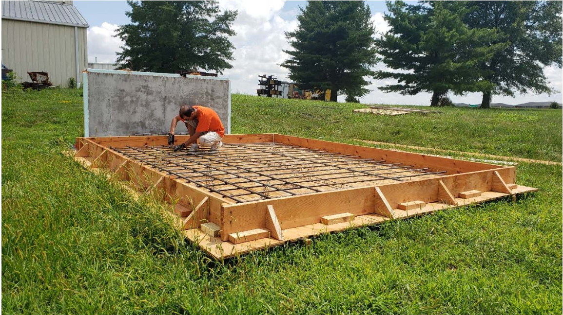
Figure 4-5: Location of the specimen in an open area next to the RTF and working on bottom layer of steel reinforcement.
