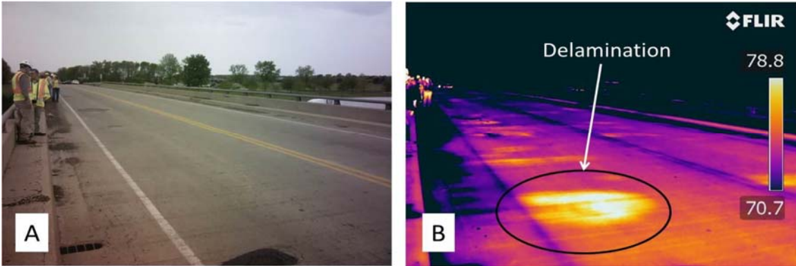
Figure 2-4: Image of a bridge deck (A) and an IR image (B) of the same bridge deck area showing a subsurface defect.
