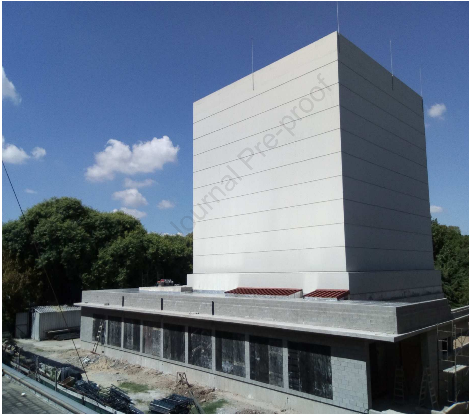
Fig. 10 Stand as of December 2019 of Accelerator development Laboratory and future BNCT treatment Centre.
