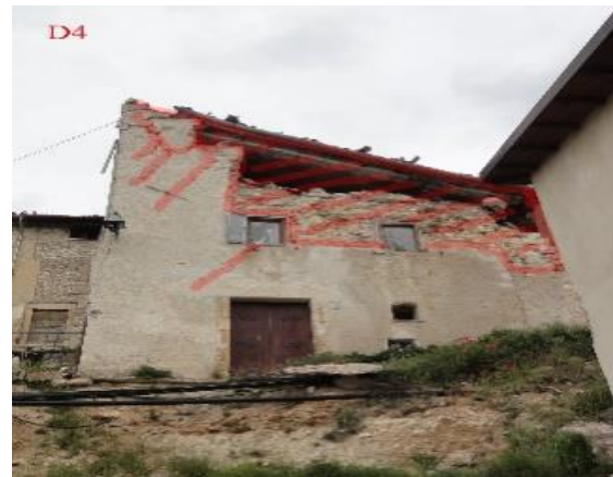
Figure 6. Structural Unite #165. Damage class D4 is assigned (EMS98).
