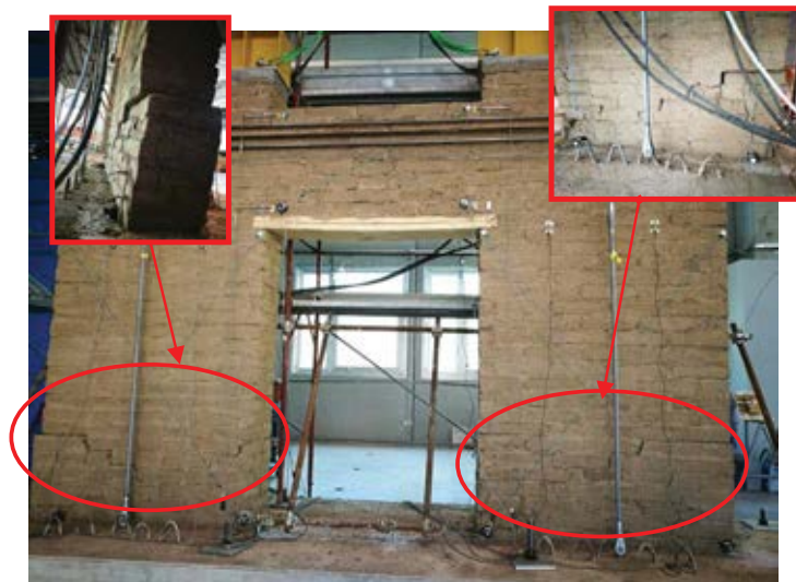
Figure 7: Damages observed on the specimen at the end of the experimental test.
