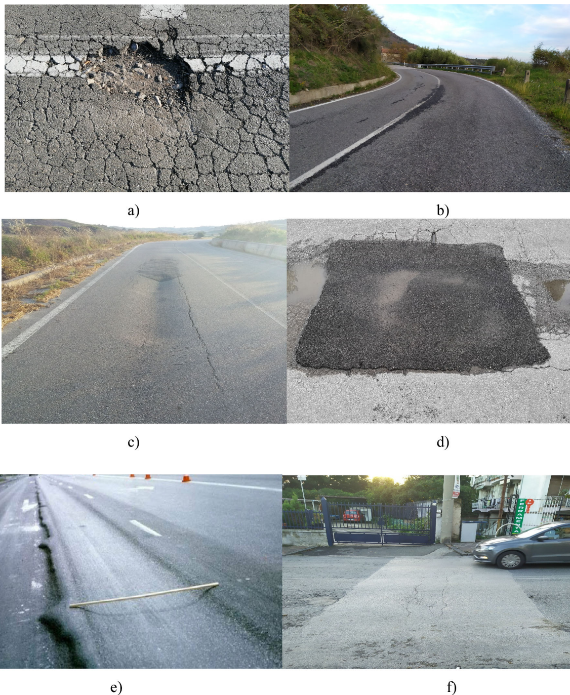
Fig. 3. Types of road distresses: a) pothole, b) raveling, c) depression, d) distress caused by local utility, e) rutting, and f) distress caused by linear utility.
