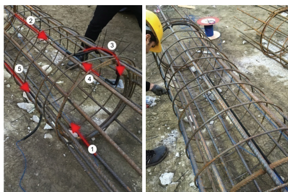
Fig. 3. The OFS installation: (a) OFS cable route, (b) anchored OFS (blu cables in the picture) and strung cable (black one).
