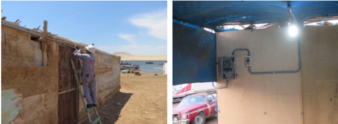
Figure 27: (a): The 500m distribution line being installed, (b): typical connection at a service point with energy meter, power limiting and main switches.
