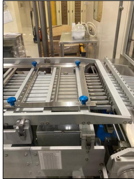
Figure 23. Start of the conveyor line
