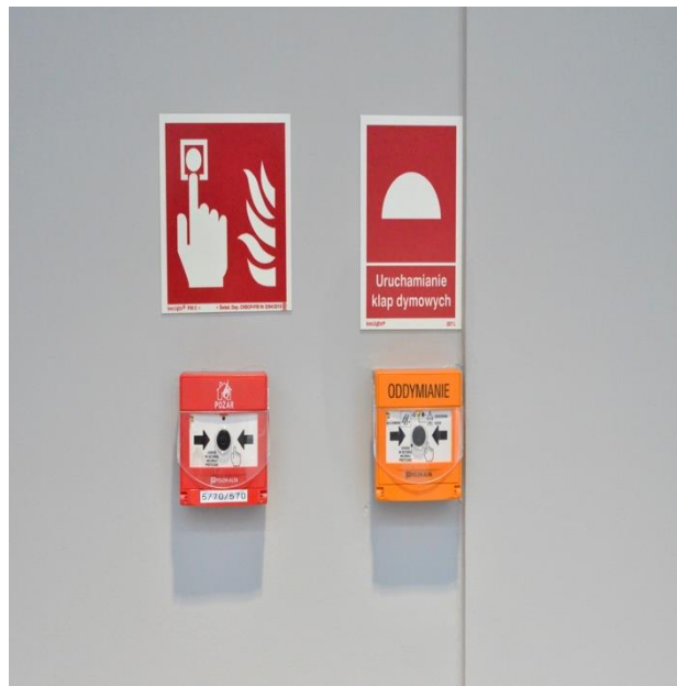
Figure 81 - Fire alarm and smoke dampers switches
