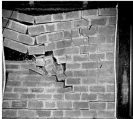
(c) Wall after test (3m height)
