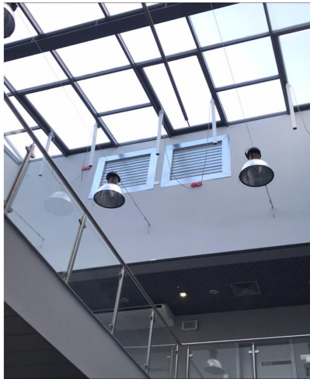
Figure 78 - Smoke exhaust fans grills closed
