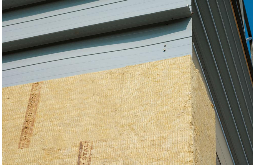
Figure 21 - An example of a static fire wall
