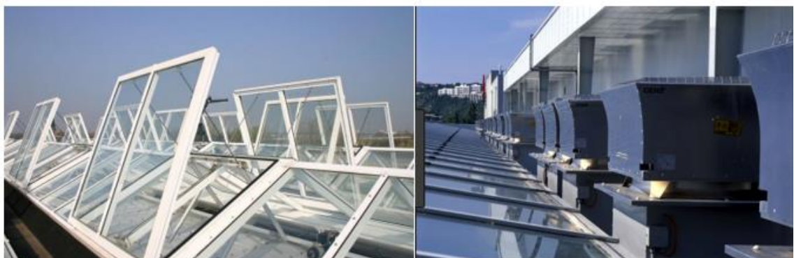
Figure 44 - Automatically opened windows and mechanical smoke exhaust fans
