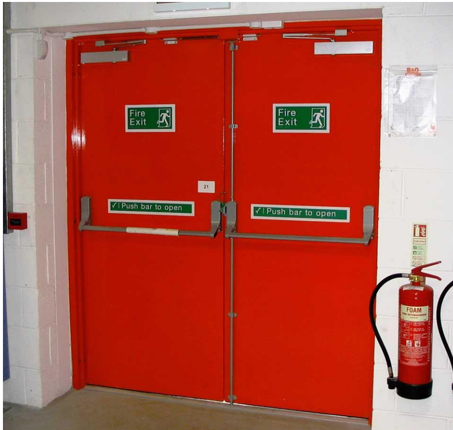
Figure 30 - An example of a fire door
