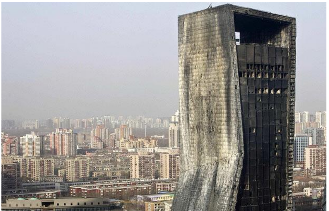
Figure 24 - Beijing Television Cultural Center after the fire
