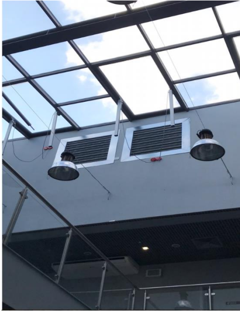
Figure 79 - Smoke exhaust fans grills open
