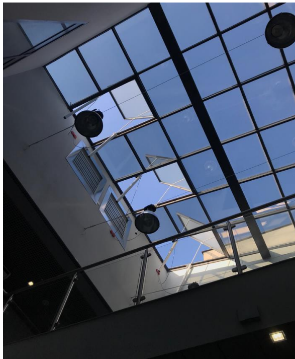
Figure 80 - Smoke dampers opened
