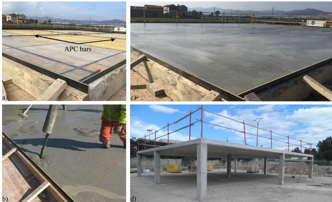
Fig. 6. Construction of the SFRC prototype: a) Installed APC steel bars; b) SFRC pumping; c) executed SFRC flat slab in the fresh state; d) SFRC flat slab after formwork removal
