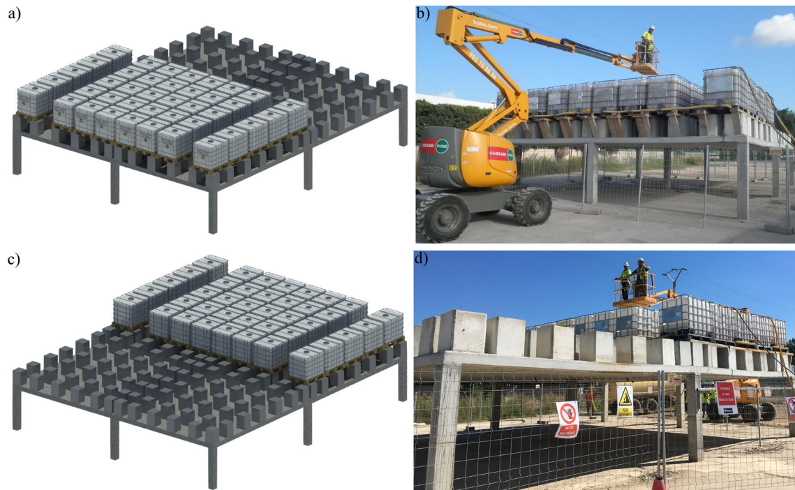
Fig. 4. SFRC flat slab under ULS conditions: a-b) ULS_I: loading of the first half of the slab (3D model and real picture); c-d) ULS_II: loading of the rest of the slab (3D model and real picture)
