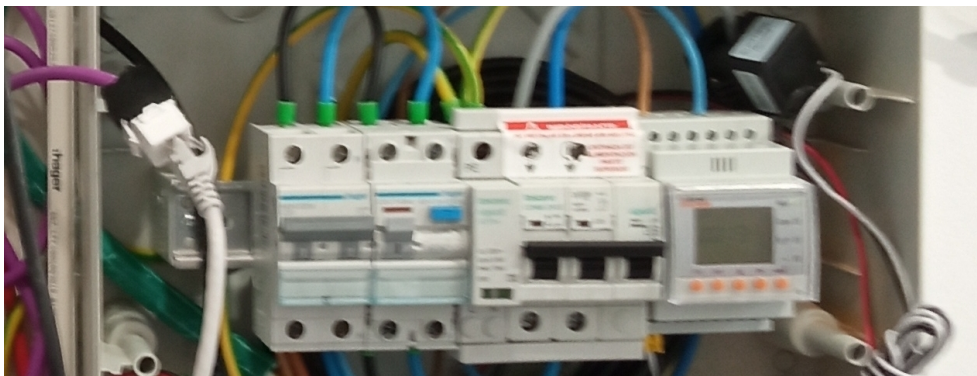
Figure 44: Meters installed in a distribution board at Ontec
