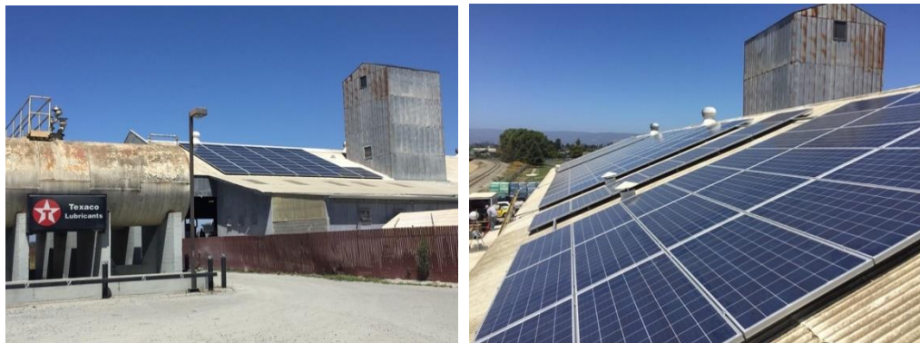
Figure 3. Rinaldi Tile 63.3kW Solar PV Installation
