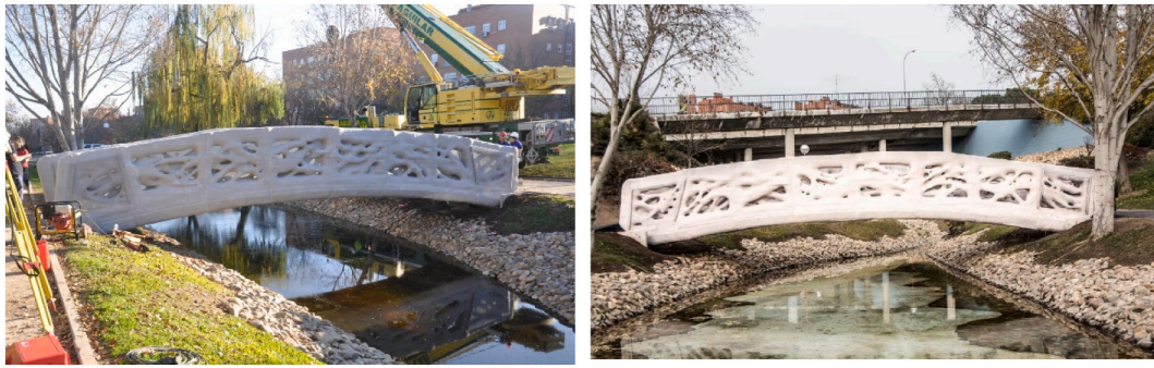
Fig. 20. a) Support and levelling operations of the footbridge and b) frontal view of the footbridge after installation.
