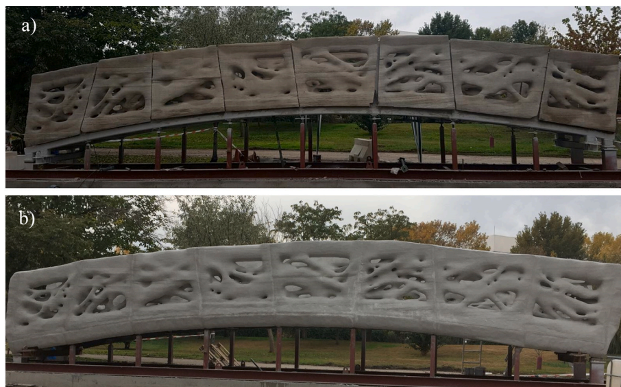
Fig. 19. a) Segments supported onto the curved steel frame and b) painted footbridge with the steel frame already embedded.
