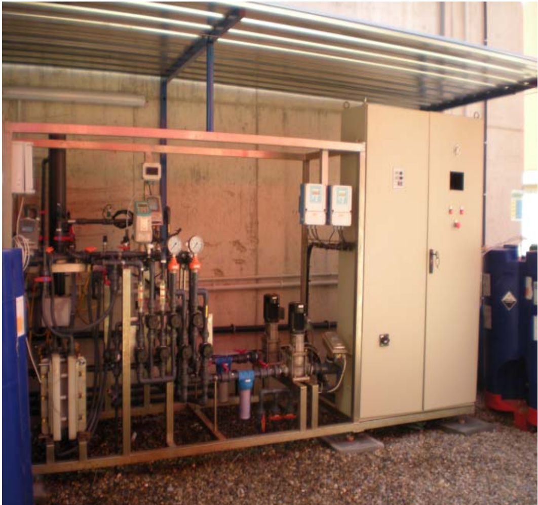
Photo 2 ED pilot plant located at the El Prat Seawater Desalination Plant.
