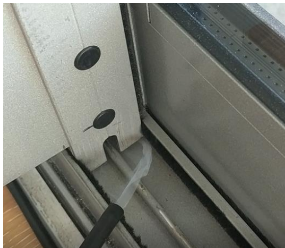
Figure 4-22 Smoke puffer testing used to visualise the air leakage paths between the sliding door and the door tracks. This was the most common leakage path witnessed amongst the tested apartments along with the exhaust fan ducting.
