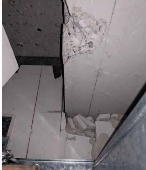
Figure 4-21 Condition of the ceiling cavity of Apartment #4, which was the least airtight apartment amongst the cohort. This building had been converted from an inner-city warehouse to a multi-unit residential building around 2000.
