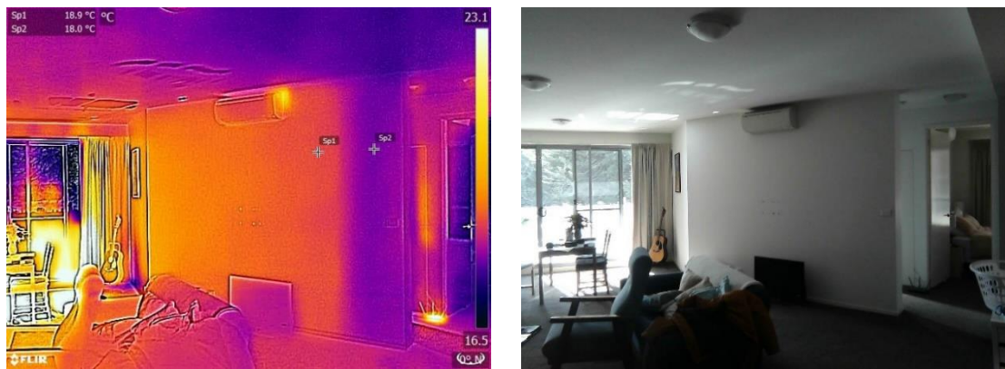
Figure 4-25 Thermographic and visual images of an internal wall in Apartment #2. The thermographic image highlights the thermal mass of a concrete column at the confluence of the living room and the bedrooms. This image was taken on 12/07/2018 at 02:10pm.
