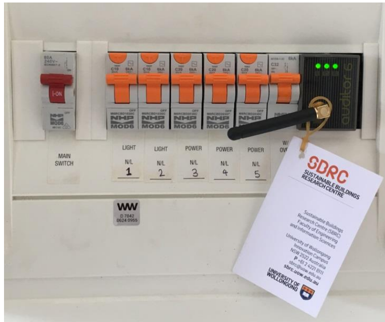
Figure 3-2 Wattwatchers Auditor 6M device installed within the circuit-breaker panel in an apartment.
