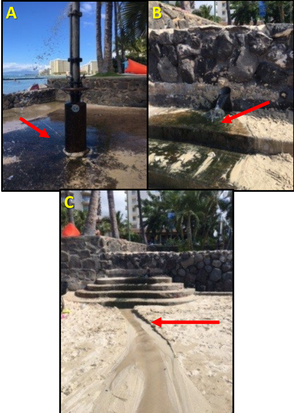
Supplemental Figure 2. Photo-documentation of Kuhio Beach Shower sampling site in Waikiki, Honolulu, Hawaii, U.S.A. Panel A is the shower platform (arrow). Panel B is the discharge pipe from the shower platform to the steps down to the beach (arrow). Panel C is the spillway from the shower discharge onto the beach. The arrow in Panel C indicates where the sediment sample was collected. Sample was collected Nov. 17, 2019 at 13:49 pm Hawaii Standard Time.
