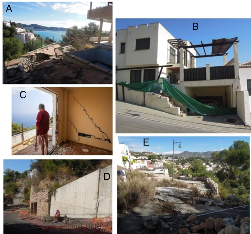
Fig. 5 Photos of damage. a Garden area of a house located in the NE extreme of Calaiza; b house in Pueblo with very severe damage; c detail of the interior of a house in Pueblo; d access road and retaining wall in Atarazanas; e access road in the Especiales site
