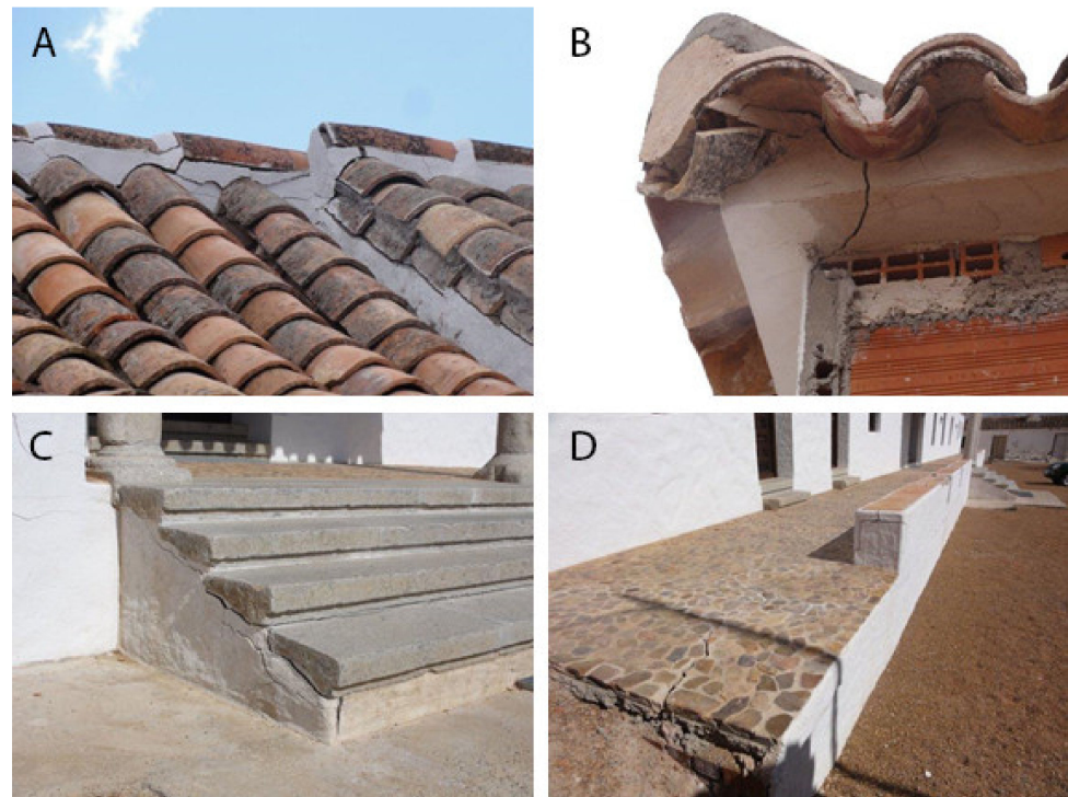
Figure 1. Photos showing the expansive nature of the mortar. (A) and (B) roof tiles, (C) and (D) paving tiles.
