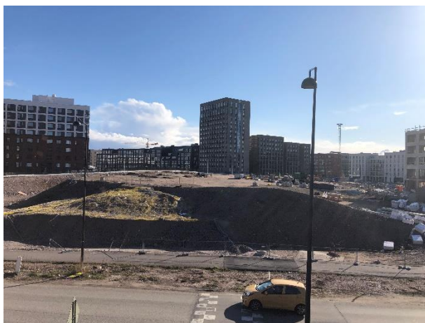
Image 12. View to a construction site where another park (Southern part of Hyväntoivonpuisto) is being built.
