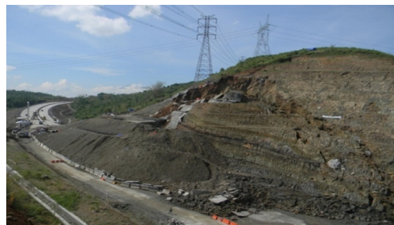
Figure 1. Slope failure on clay shale at STA 19+250 Semarang-Bawen tol road during construction (Himawan, 2013)
