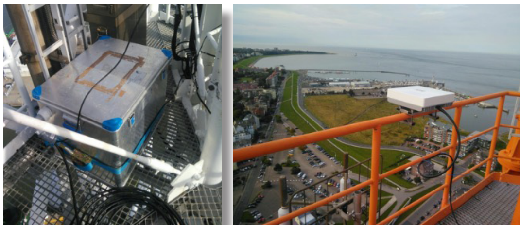
Fig. 9.2: ZargesBox containing all modules for the land station (left) and the antenna mounted approx. at a height of 90m a.s.l. in the direction of the German Bight (right); photo: P. Sprich, WSA
