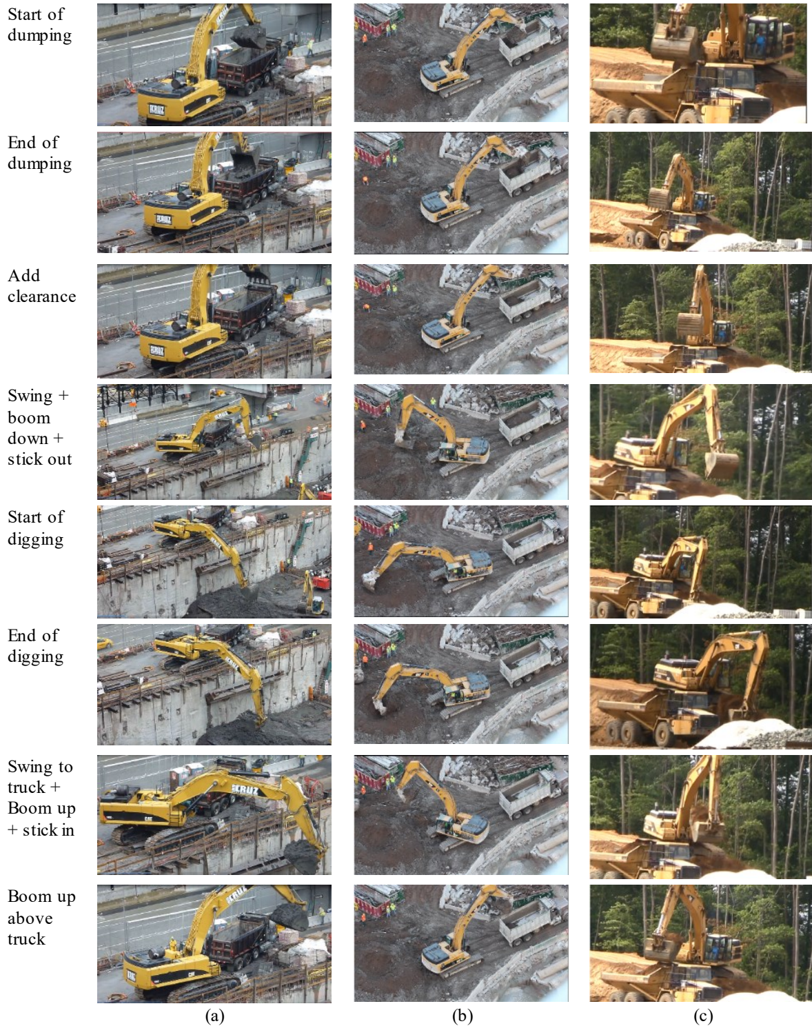
Figure 3.1 Snapshots of excavators loading trucks: (a) The digging is at a very low level forcing the boom and the stick to extend almost to their maximum angles, (b) The excavator is in the middle between the digging area and the truck, (c) The truck is at a level lower than the excavator. (Hammad et al., 2014b)
