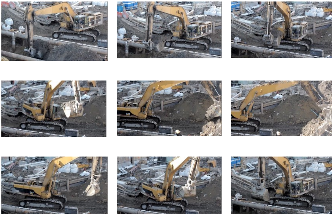
Figure 3.2 Unsafe situation because of underground pipes (Hammad et al., 2014b)
