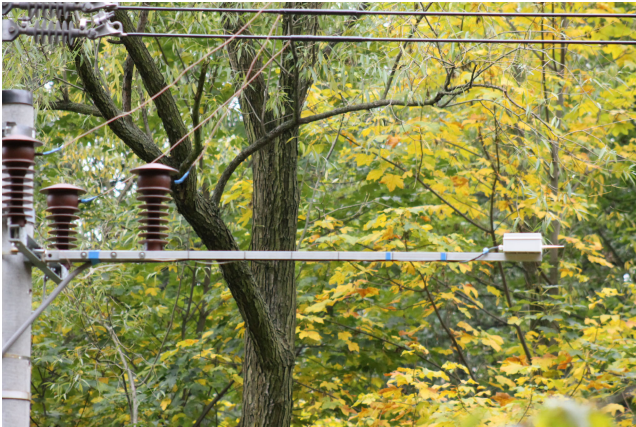
Fig. 2. Antenna mounted under overhead power line.
