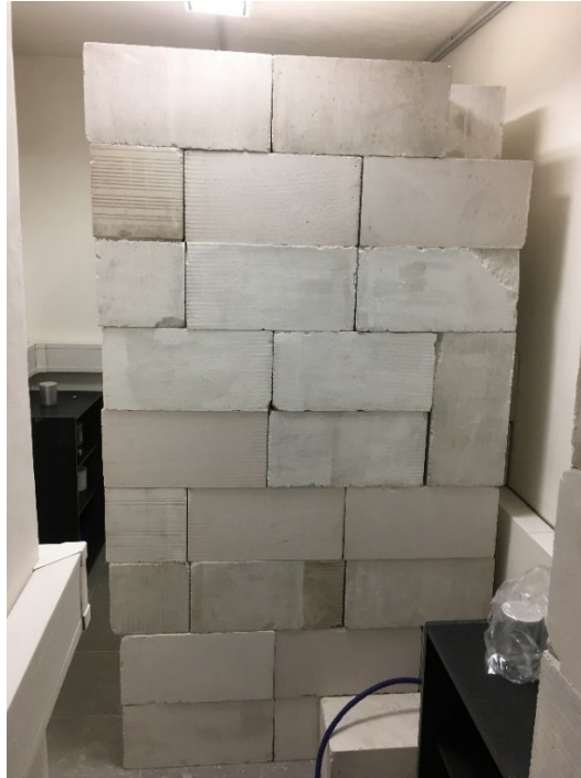
Figure 3.6: Shielding at VŠB-TU Ostrava; the wall was created with YTONG blocks to shield incoming neutrons.
