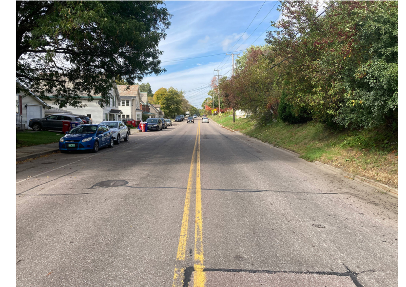
The painted stripe separating the shoulder/bike lane is not well maintained as seen in this image.
