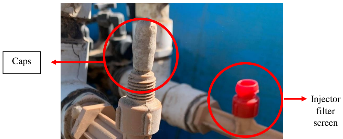
Figure 1.3 Air is injected to water flow using venturi air injector and injector filter screens.
