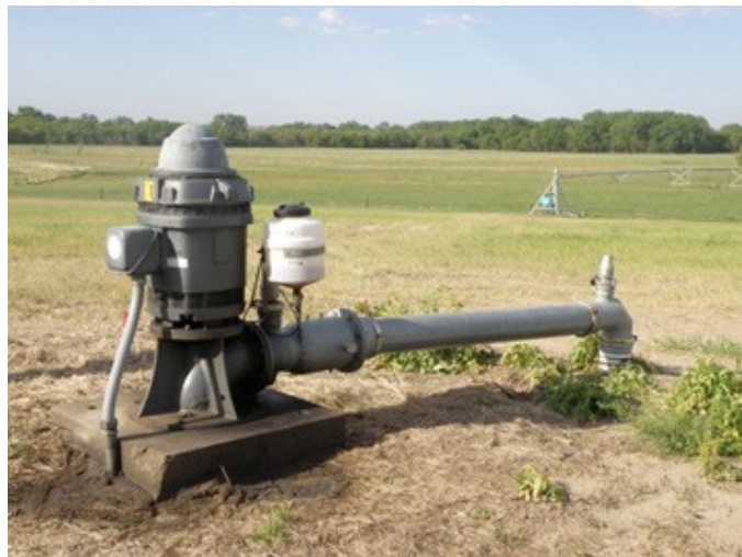
Figure 14. Electric motor for pumping irrigation water.
