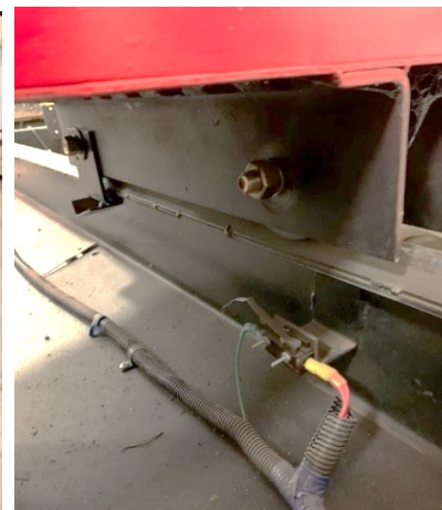
Figure 12: Example setup of a limit switch on the weight box rail. The attachment attached to the weight box will advance toward the switch and trip the system to stop motion of the box.
