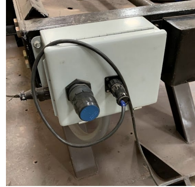
Figure 6: Image of the front electrical box, which encases the second J1939 connector for the attached tractor, load cell connector.
