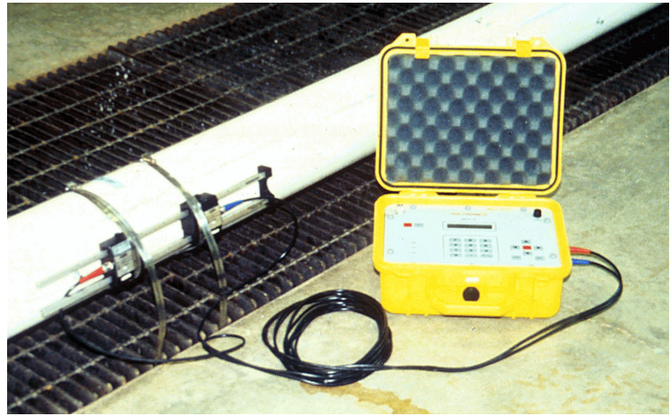
Figure 3.13. Clamp-on ultrasonic meter installed on a pipeline.
