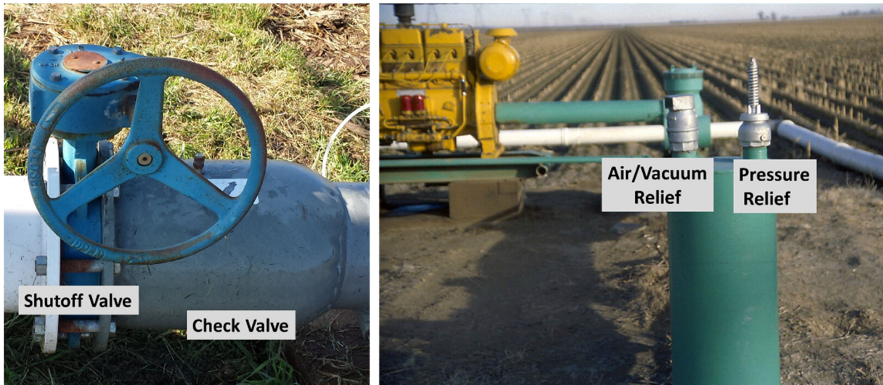
Figure 8.6. Irrigation pipeline protection valves.
