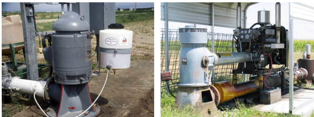
Figure 8.15. Pumping plants including a well with a vertical turbine pump and a power supply: electric motor (left) and internal combustion engine (right).
