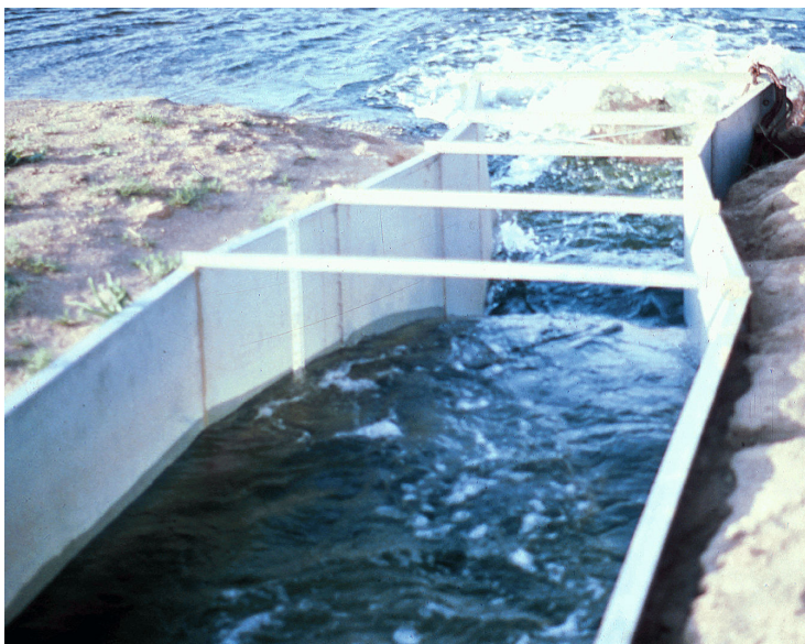
Figure 3.19. A Parshall flume to measure open channel flow.
