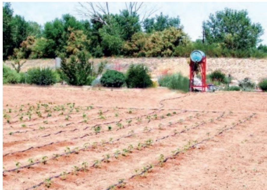
Figure 14.6. Example of an arrangement at the control station for a microirrigation system.
