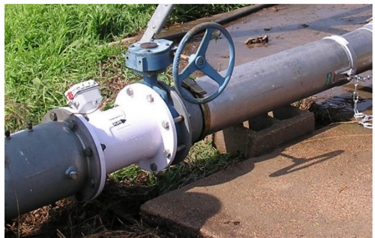
Figure 3.15. Electromagnetic flowmeter installed in the field.
