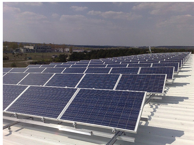
Fig. 6 PV system, FRoSTA company (a photograph provided by FRoSTA)
