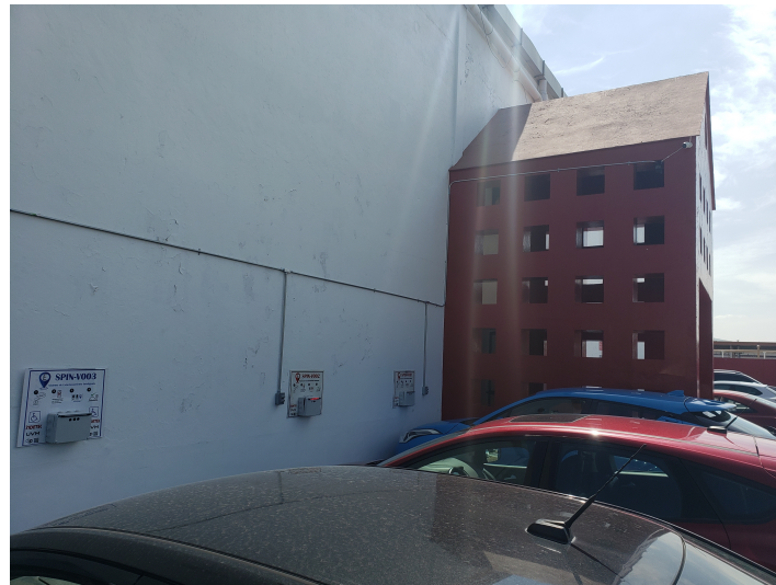
Figure 20. Three SPIN-V Installed in UVM.
