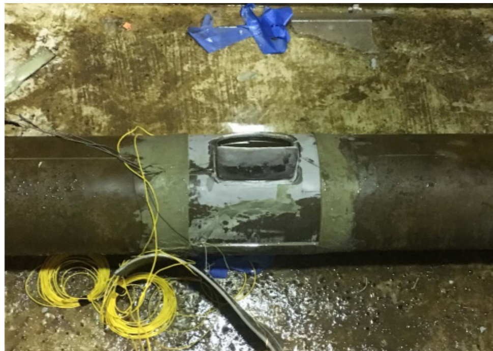
Figure 25. Typical composite pipe that is repaired with CompositSleeve™ sample after pressure testing showing the attached optical fiber sensors (Reprinted/adapted with permission of Dr Chris Alexander. Copyright 2018 ASME & Chris Alexander. Source: Ref. [377]).
