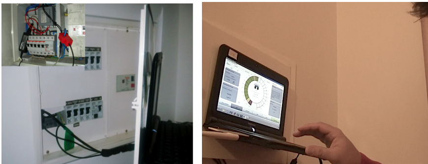
Fig. 1. System installed in the main power feed (left) and a householder interacting with the eco-feedback (right)
