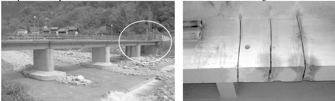
Figure 1. General view of Dogna Bridge (left) and detail of damages D1-D6 (right).
