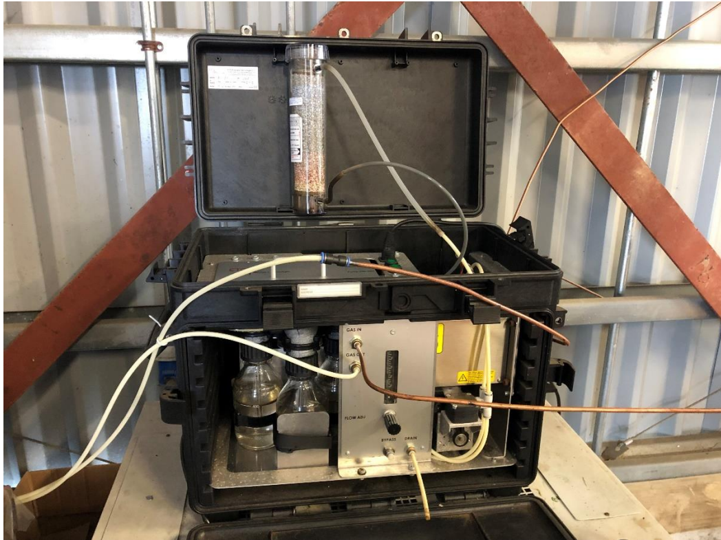
Figure 3.12 Scrubber with moisture capturing DRIERITE material. Discolouration can be seen where material has absorbed moisture.
